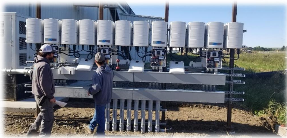
480V SolarEdge Inverters
